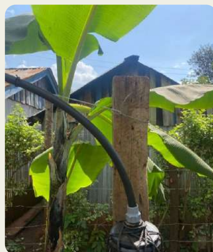
Pipe connection to filter
